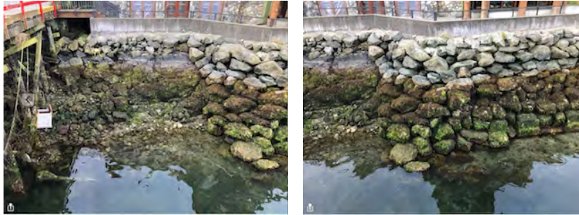
Riprap and bedrock showing intertidal zonation views in front Whiskey Landing Phase I
