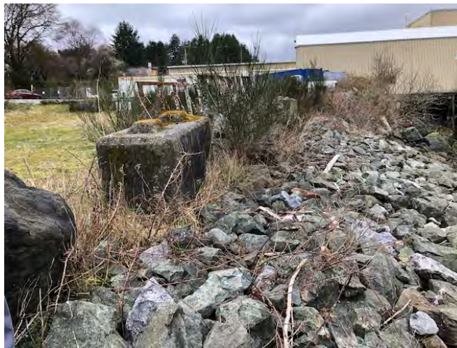
View north along HWM at T-2 showing upper riprap and riparian zone.
